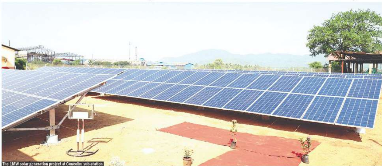
The 1MW solar generation project at Cuncolim sub-station
